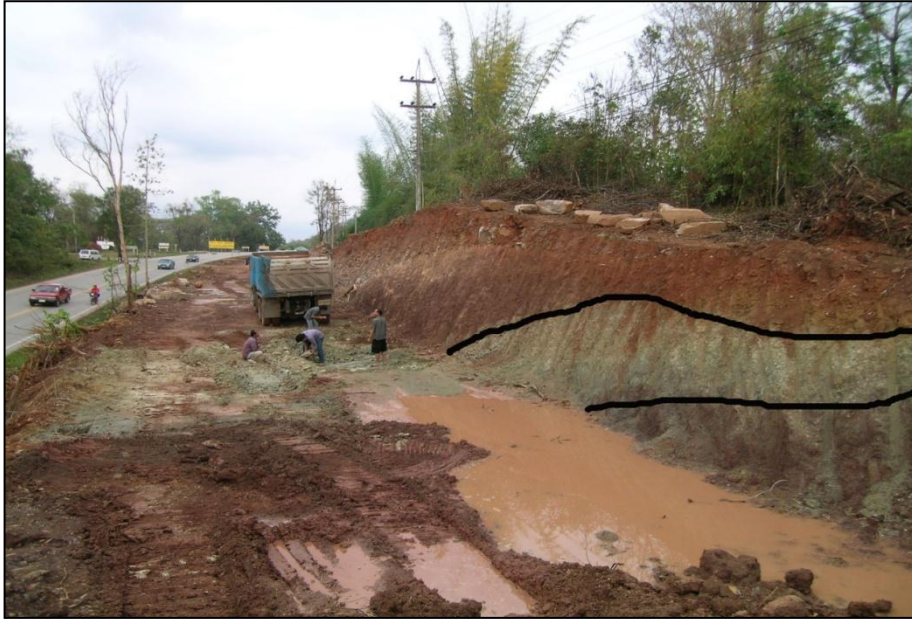
Figure 3.2 Fossil bed of Phu Phan Thong locality (black line), Nong Bua Lamphu Province, during the improvement work of road 210 in 2003
