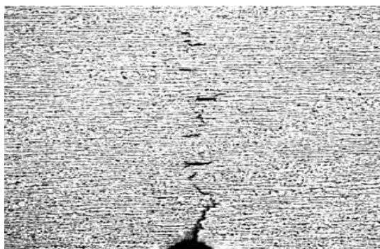
Figure 2.12 Hydrogen embrittlement corrosion
